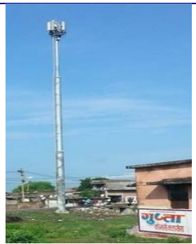
Pole type Reliance Jio tower
